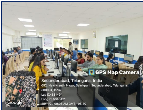
ROOM N21A: LAN SETUP
