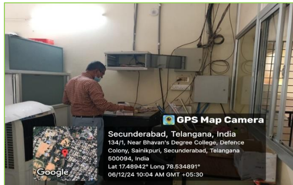
RECEPTION ROOM: LAN SETUP
